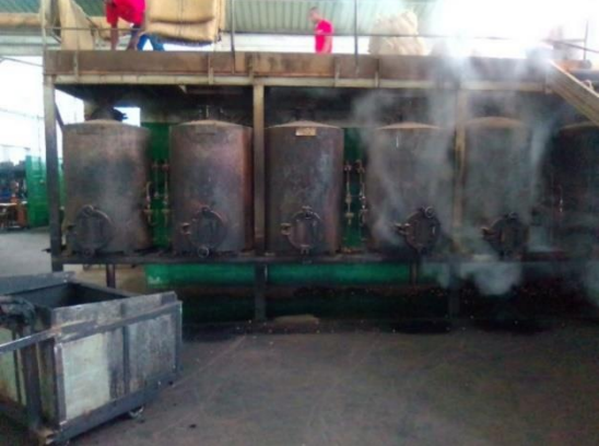
Picture 8.2. Ovens Used for Steam Heating
